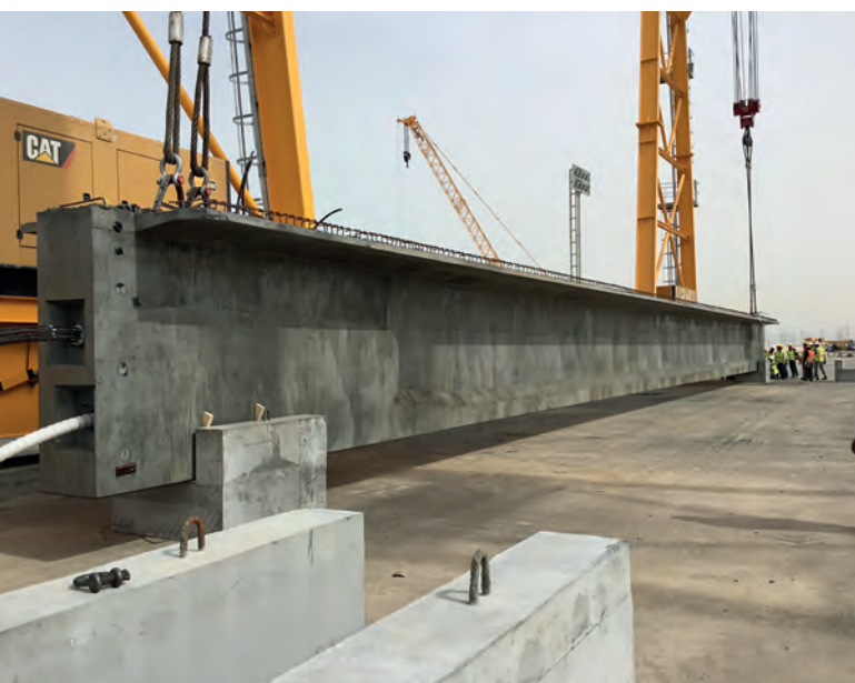
The elements are produced post-tensioned. Eight elements can be produced daily. For all bridges a total of 820 girders are required.
