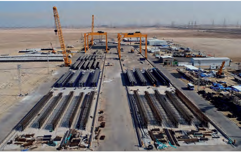
9 of the bridges are constructed with precast concrete elements, which are produced on a local precast yard by using of moulds from Tecnom.
