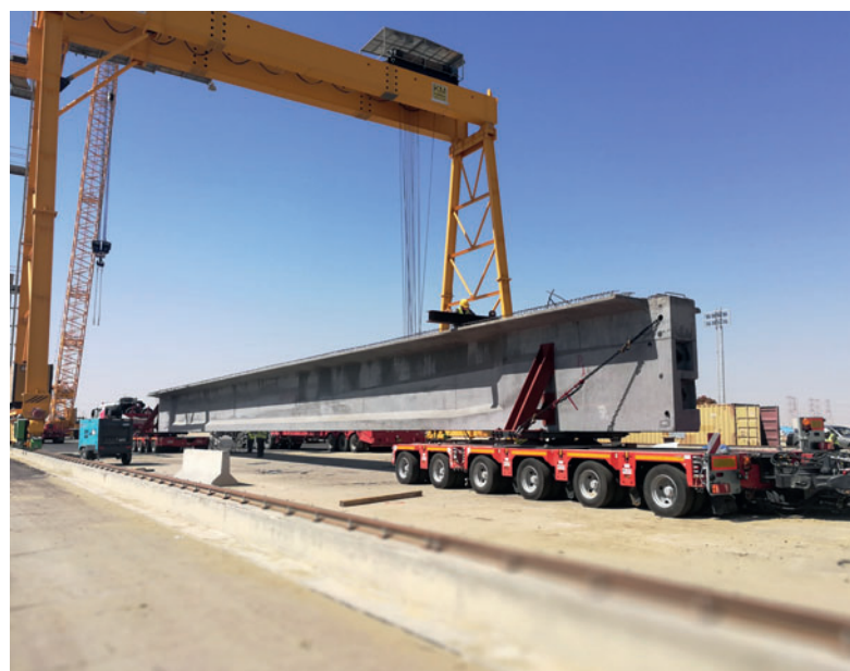
Due to the convenient location of the production yard, which is placed in the middle between the 2 furthest construction sites, the transport ways have been minimized to 20 km max.
