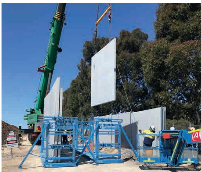
Noise-Controlling wall panels from BGC Precast are installed on the North Link Motorway, near Perth in Western Australia. (Credits: BGC)
