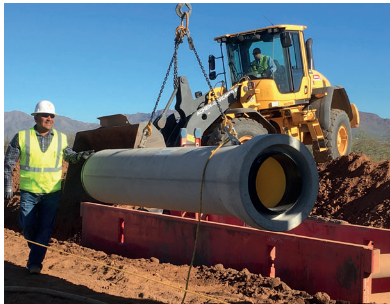
Installation of Perfect Pipe in Pima County, Arizona, in 2017: a considerable number of pipe DN400 (16") was laid in open trench under real installation and usage
