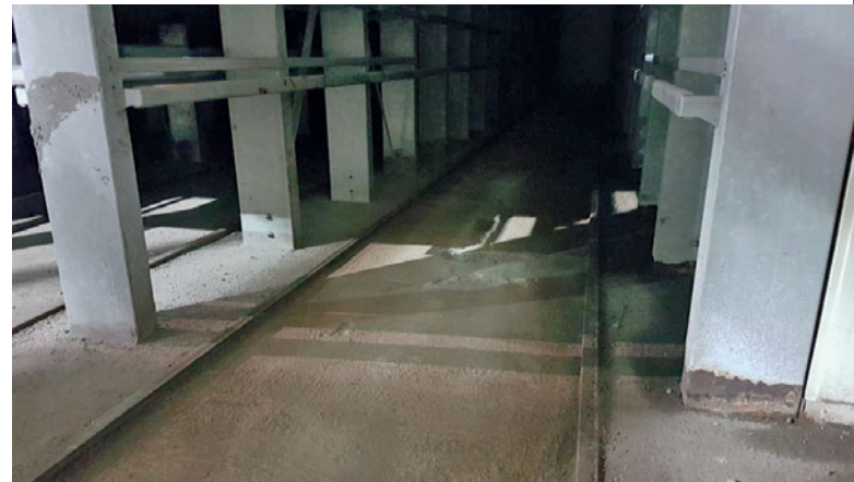
Typical effect of condensation: columns closer to the chamber's center are dry and free of corrosion while those located at the perimeter (right) have corroded at the bottom
