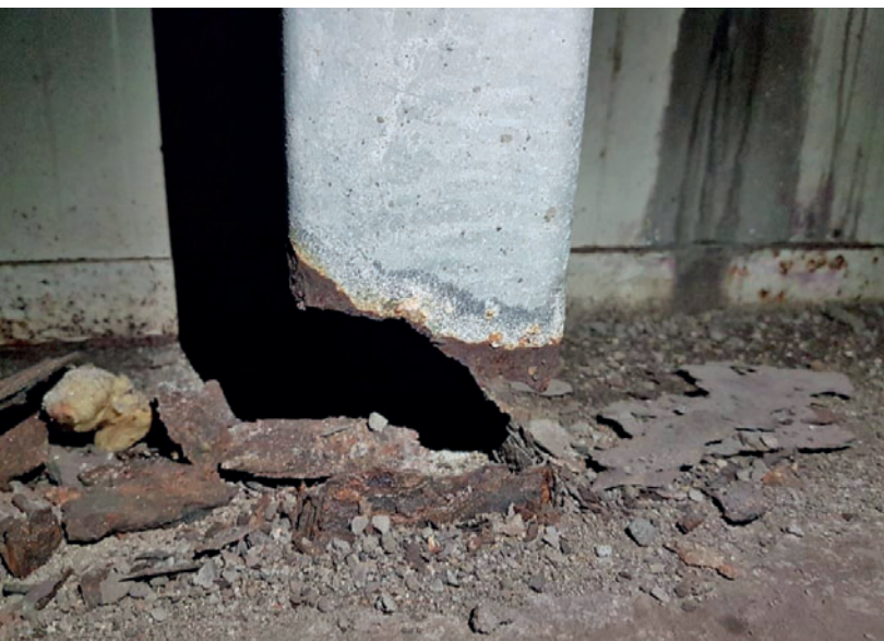
Column corroded due to condensation. This completely corroded lower column portion is only held in place by the rest of the rack system and requires immediate replacement
