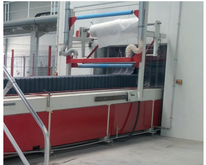
A Mega 6000 Duo aging machine from SR-Schindler was integrated as a bypass system on the dry side for the refinement of the concrete products.
