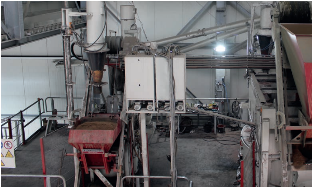
Two compulsory mixers from the Hess SM series were installed on a mixer platform for the production of the concrete.
