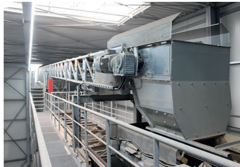
The core concrete aggregates are transported by a new conveyor belt from the adjacent original hall.
