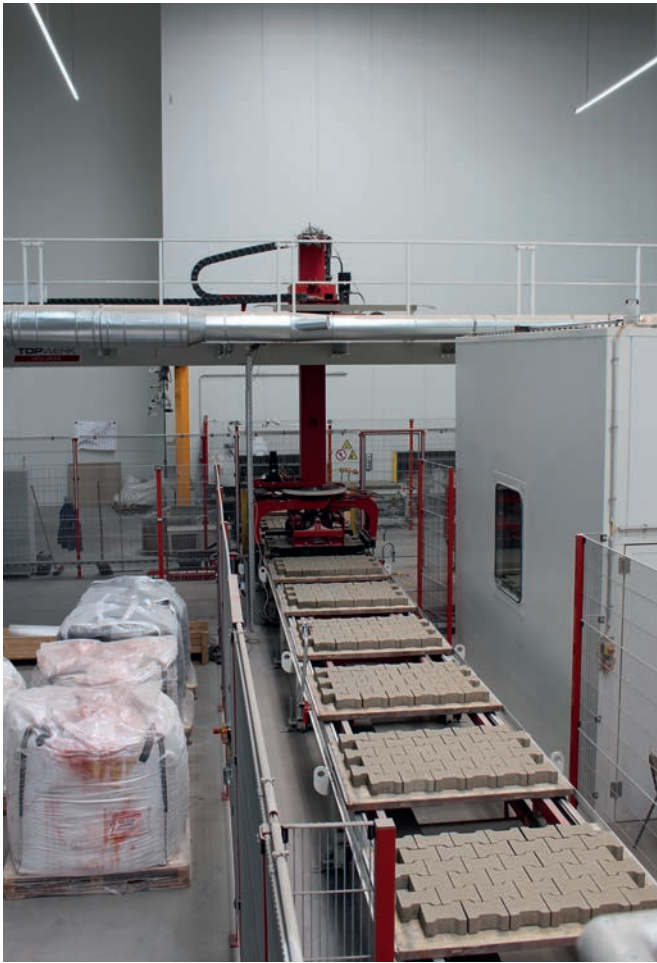
The first cuber is located behind the bypass. This either releases the stones or supplies the refinement machine from SR-Schindler with concrete products.
