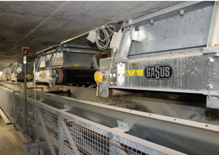
With a capacity of 3,000 kg/min the individual aggregates are weighed additively by dosing belts onto a weighbelt
