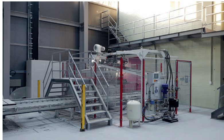
A double washout unit is installed in the transport system on the wet side.
