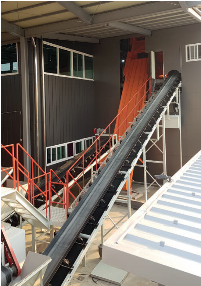
A dosing belt under the bunkers weighs the aggregates for the core concrete and fills them into the lifting bucket.
