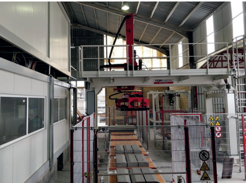
Dry side with Topwerk Electric cuber
