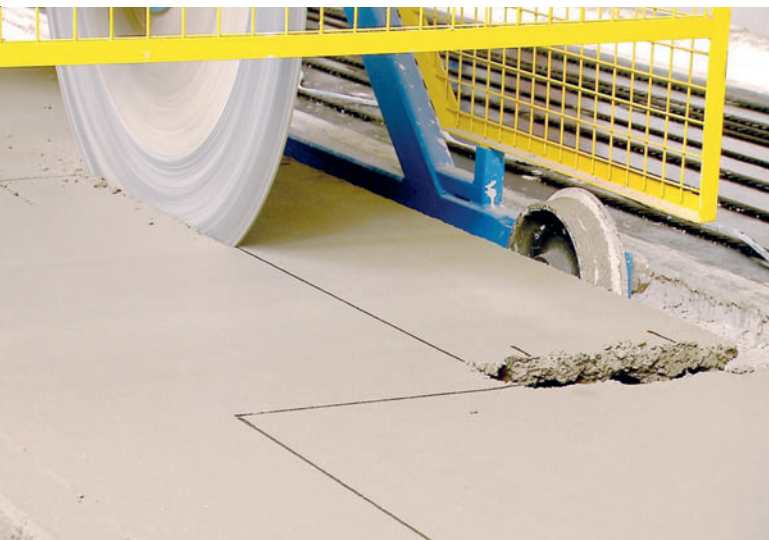
With the fresh concrete saw hollow core slab can be processed directly after the finishing process without any problems.
