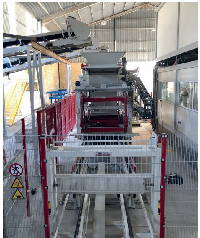
Multimat RH1500-3MVA de Hess
