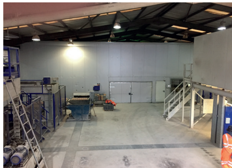
Insulated transfer car area including elevator and lowerator. Double-door for equipment access, personnel door and large window.
