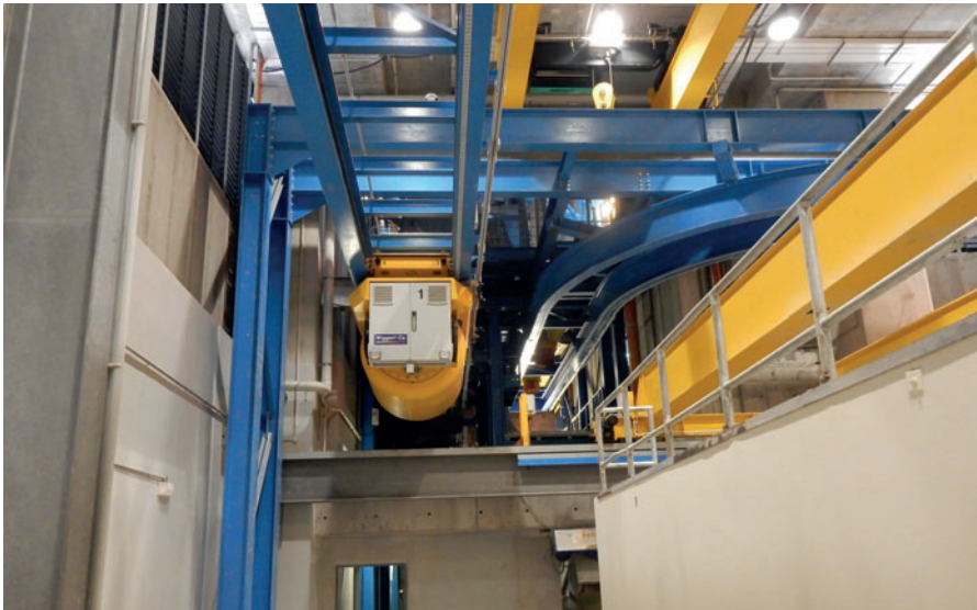
Even the fresh concrete is delivered automatically to the production lines by means of various bucket conveyors.
