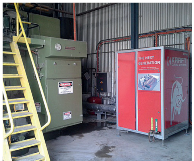
The vapor generator is not only a money saver but also a space saver - pictured here alongside the steam boiler that it replaced.
