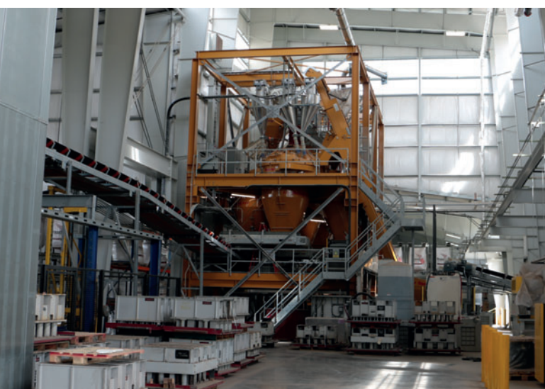
A central raised platform holds the entire mixer operation for both plants
