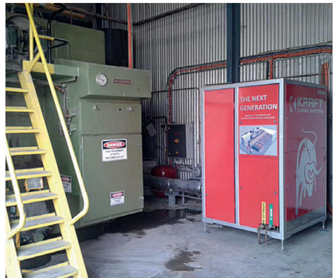
The vapor generator is not only a money saver but also a space saver - pictured here alongside the steam boiler that it replaced.
