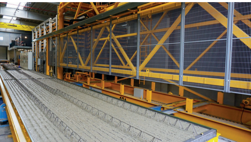
Positive customer feedback has already been received: thanks to the new plant, Isodal is now producing lattice girder floors with accurate dimensions and a perfectly smooth surface.
