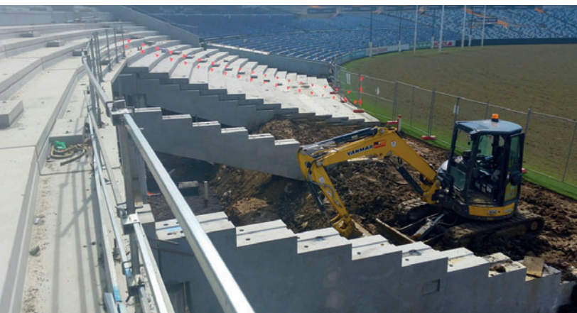
Already, two stadiums have been equipped with the stadium slabs produced by the new slipformer.
