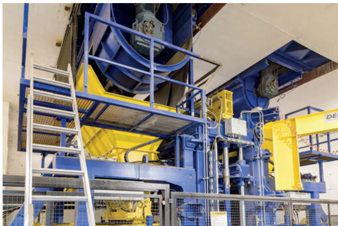
The concrete is discharged from the block making machine's storage silo into the core concrete feed box.
