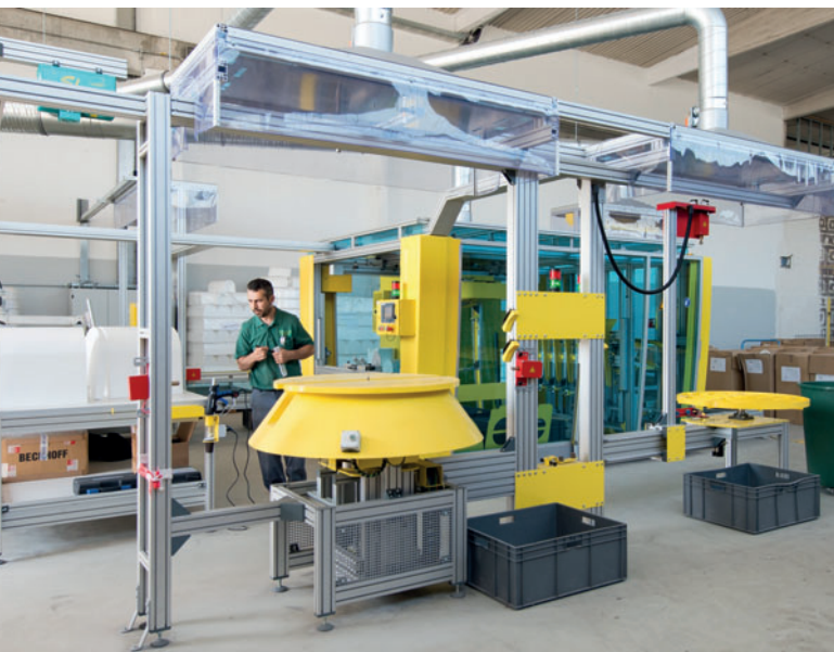
Globally tried and tested production technology now used at Beton Kemmler - image shows the EPS cutting technology
