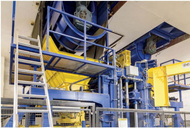
The concrete is discharged from the block making machine's storage silo into the core concrete feed box.
