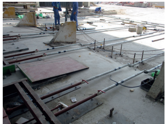
On-grade installation of the ThermalCure hot water supply and return lines and connection to the casting beds.
