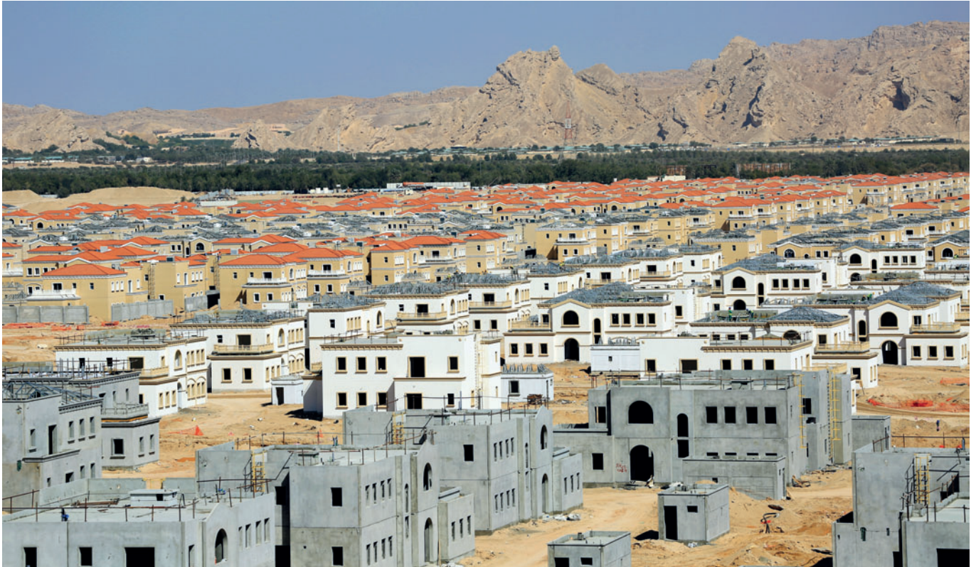
An example of Hi-Tech's scope of precast concrete villa supply and an excellent example of the benefits of precast concrete's advantages in terms of speed of erection, quality, efficiency, versatility and durability.
