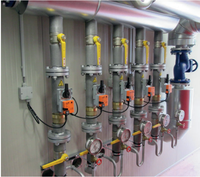
A total of 6 hot water supply lines supply 95°C hot water to a total of 6 casting beds. Each line includes an automatic valve with (orange) actuator. One main return line for all 6 casting beds returns water back to the water heater for reheating.
