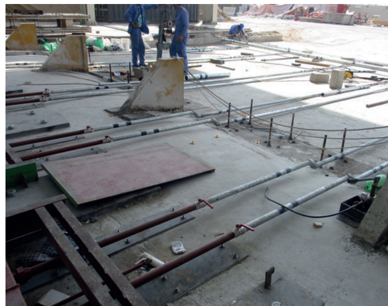
On-grade installation of the ThermalCure hot water supply and return lines and connection to the casting beds.
