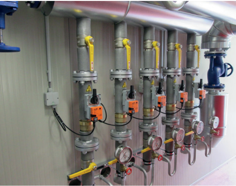
A total of 6 hot water supply lines supply 95°C hot water to a total of 6 casting beds. Each line includes an automatic valve with (orange) actuator. One main return line for all 6 casting beds returns water back to the water heater for reheating.
