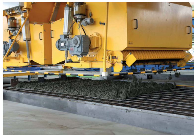
An automatic concrete spreader places the fresh concrete precisely and at a steady rate on the pallet.
