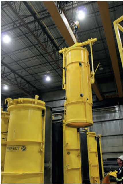
A crane transports the formed liner (with pallets) to the formwork mold and sets it down over the shrinkable mold core
