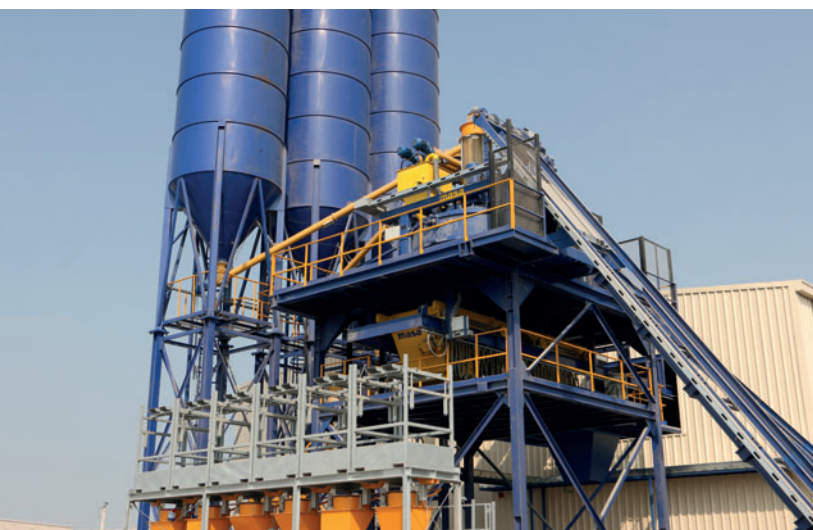
Masa mixing tower: Below the concrete mixers you will find the Masa double bucket conveyor
