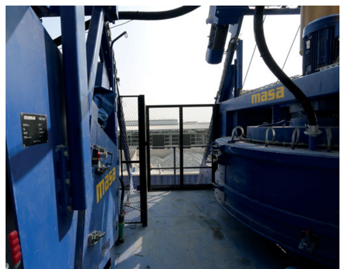
The new plant is equipped with two Masa concrete mixers: Masa mixer PH 2000/3000 (right) and Masa mixer S 350/500 (left)
