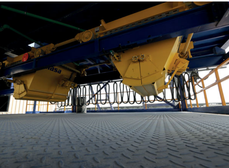
The ready mixed concrete will be transported to the block making machine by a double bucket conveyor
