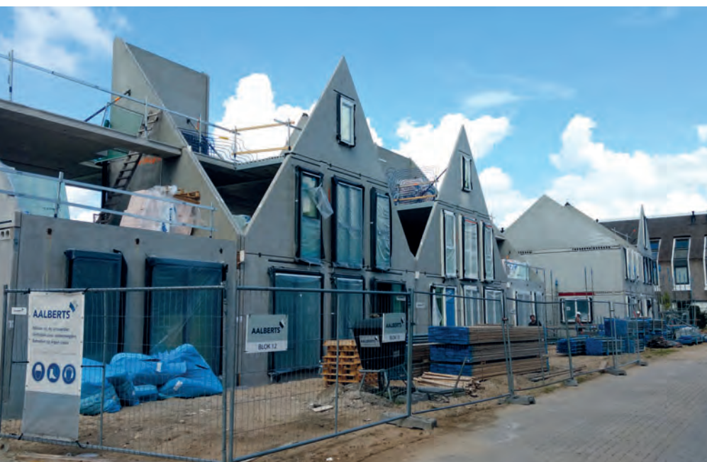
The precast concrete construction method is now also very popular in private residential construction. A special assembly concept enables Geelen Beton's customers to realise buildings within the shortest time.
