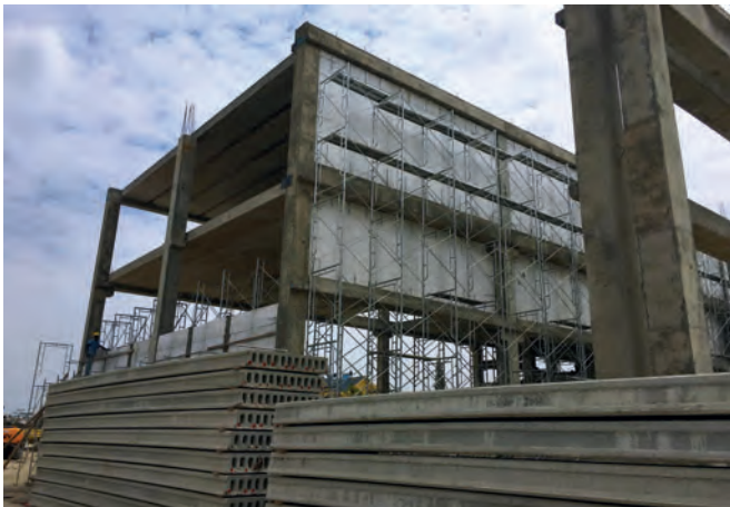
Using plant and mould systems from Echo Precast Engineering and Tecnom, Boleyn Magic Wall Panel is manufacturing hollow core slabs, sandwich walls, columns, beams and other structural precast concrete and special elements.
