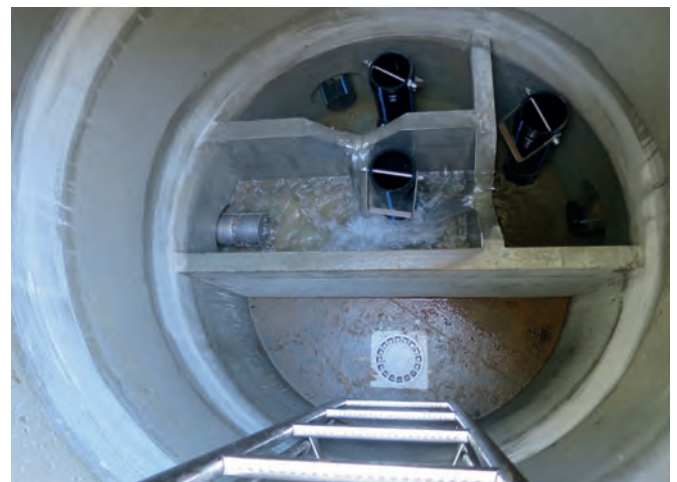
View inside a DN1500 concrete water chamber tailor-made by Wyss AG, with multiple inlets and 4 chambers at the water catchment site in the municipality of Vitznau, on Lake Lucerne.
