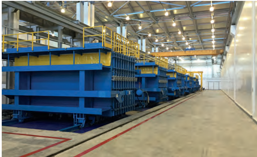
Solid walls and slabs are manufactured in the smallest space using a total of 18 battery moulds.
