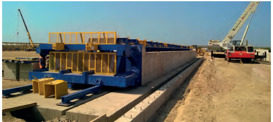
The 40 m mould was installed in the vicinity of the construction site. It can be used independently of location, since it has a self-stressing system.
