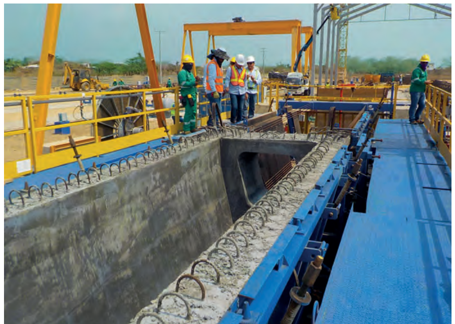
A vibration and heating system ensures steady compaction and curing of the concrete used. V girders in three different lengths, weighing up to 85 t, were produced for the "viaducto Gran Manglar", the longest road bridge in Colombia.
