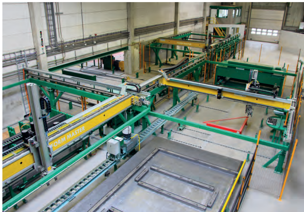
The core of the renovated Voorbij Prefab plant is the Form Master shuttering and deshuttering robot. Infinity Line® makes it possible to shutter without leaving gaps and without using polystyrene elements, while at the same time reducing the number of shutters required to a minimum. For the first time this system is applied for solid wall shutters.
