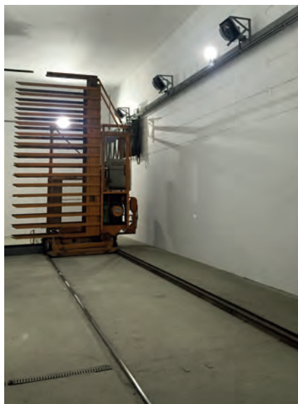
Due to the air distribution in the transfer table aisle, this area and the finger car remain dry. No condensate or mist forms that could result in a possible failure of the finger car distance measurement, which is carried out by lasers.
