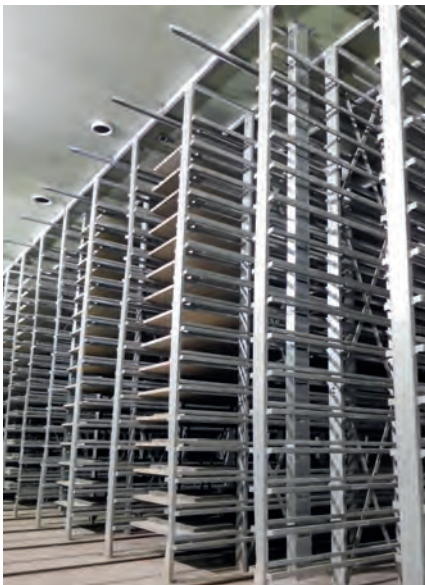
Air distribution lines inside the chamber to regulate air distribution and limit air velocity to less than 1.00 m/s.
