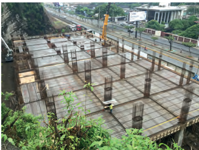
In August this year a five-storey car park was constructed for the Catholic University of Guayaquil. An addition of two more levels is planned.
