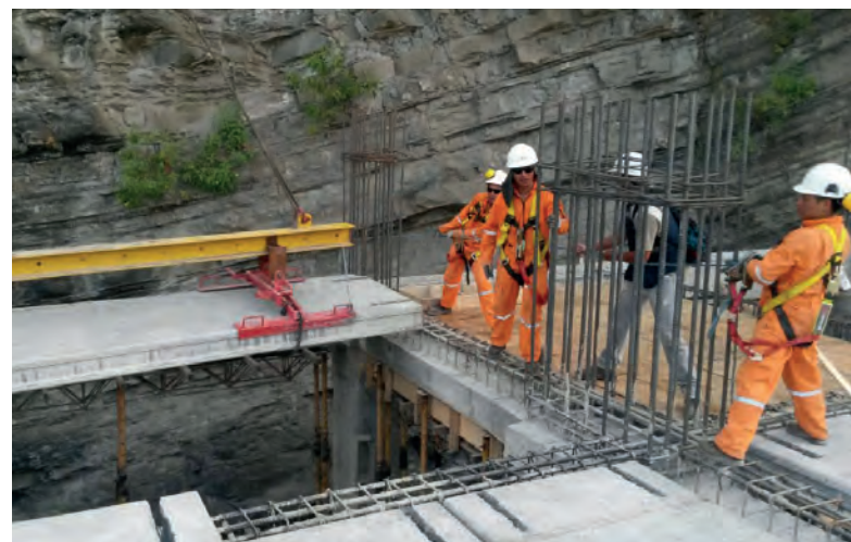
EPCE transported hollow core slabs, each 8 m long and for a total surface area of 10,000 m 2 , from Riobamba to Ecuador's largest city.
