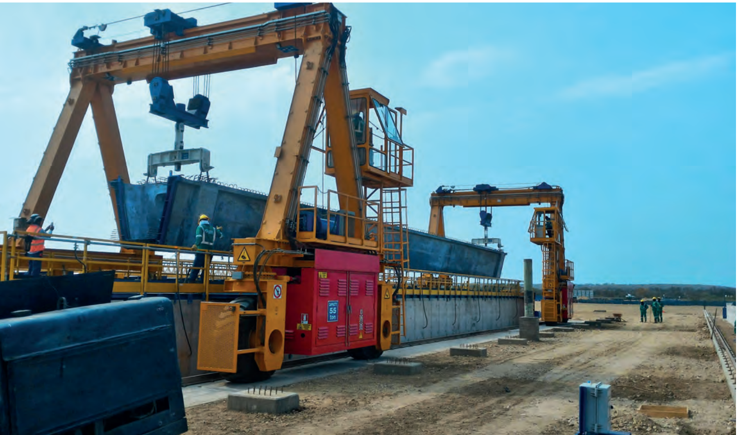
Two gantry cranes load a total of 387 concrete elements on to special HGVs, which transport them to the construction site.
