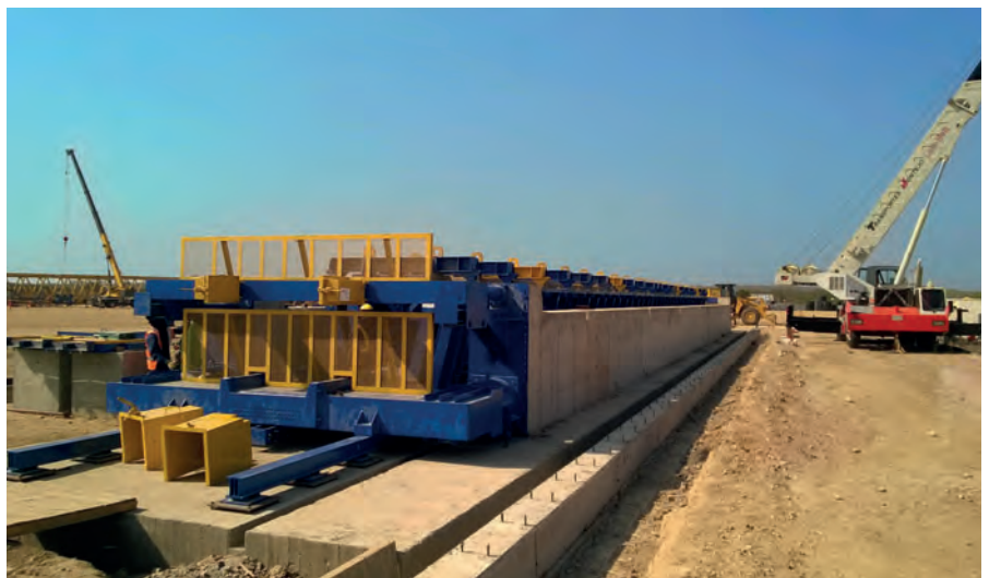
The 40 m mould was installed in the vicinity of the construction site. It can be used independently of location, since it has a self-stressing system.
