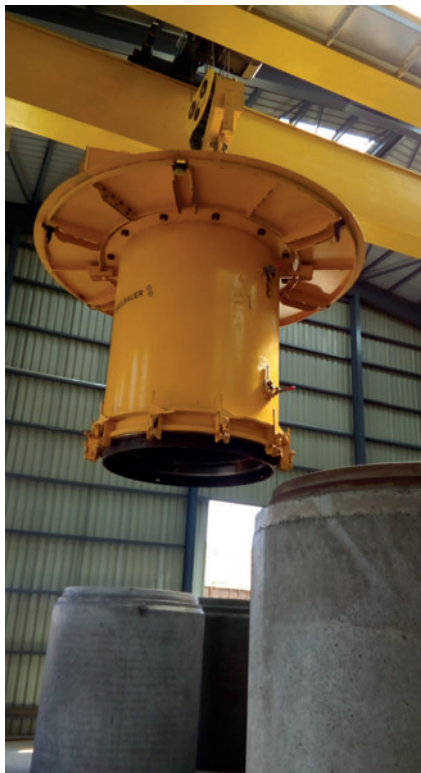
The pipe that has been freshly cast is brought to the setting area using an indoor crane.
