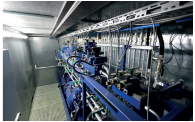
View inside the Masa Hydraultainer
