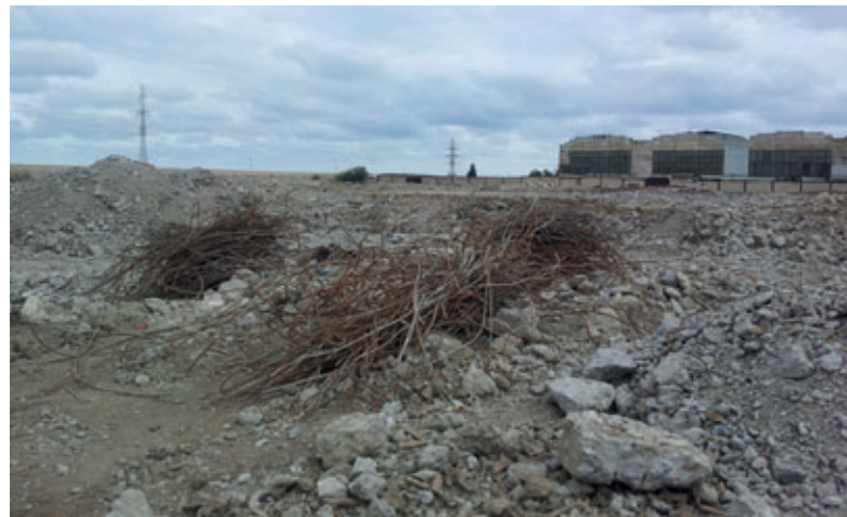
The future "Star CP" production facility terrain during the first site inspection
