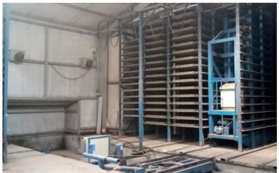
Thanks to the circulation of air in the transfer car area, both this area and the transfer car remain dry. No condensed water forms on the ceiling and there is no mist formation, which could lead to failure of the finger car's laser distance measuring system.
