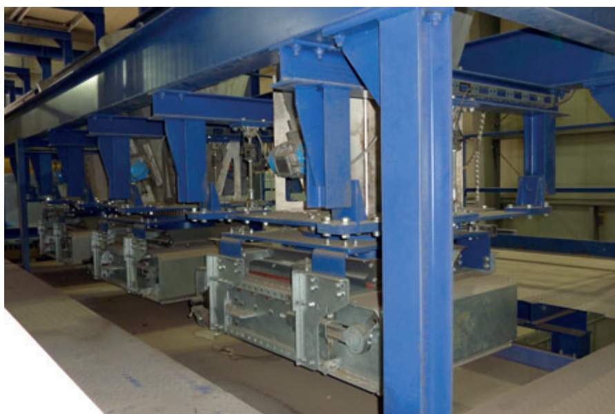
The conveyor belts can be swiveled by approximately 30 degrees to the left or right from the center position during dosing of the colored concrete
