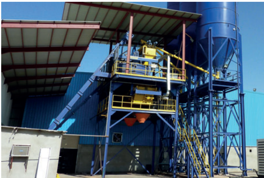
View of the Masa mixing tower: The cement screws feed cement into the cement scales of the Masa mixers S 350/500 and PH 2000/3000
