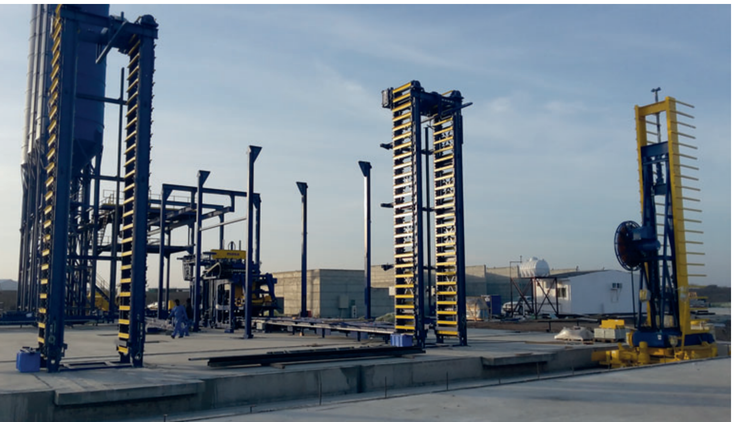
The installation work is progressing: elevator, lowerator as well as the Masa finger car are assembled.
