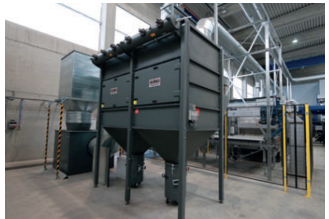
Rotho central dust extraction unit
