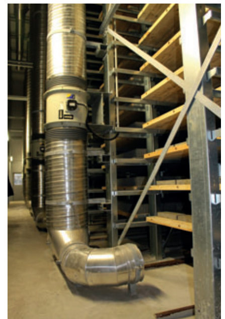
The Rotho circulation system generates a uniform climate
