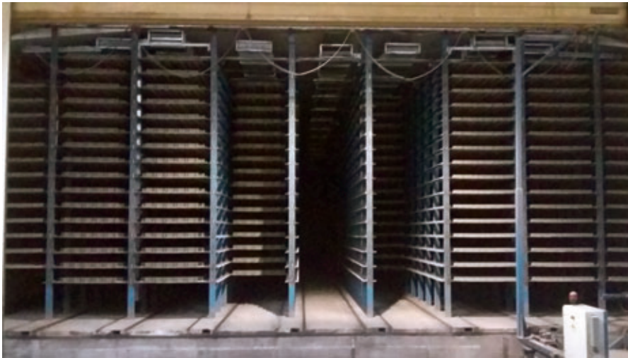
The galvanized supply and return ducts are mounted above the rack system. They don't take up necessary space. The floor is dry from front to rear in every corridor despite a humidity of 95 %.
