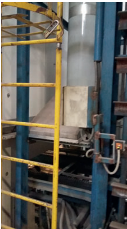
One of two heated hoods, installed between the lowerator and the exterior wall of the chamber, which prevents the escape of warm, moist air from the curing chamber and thereby prevents condensation dripping onto the fresh stones.
