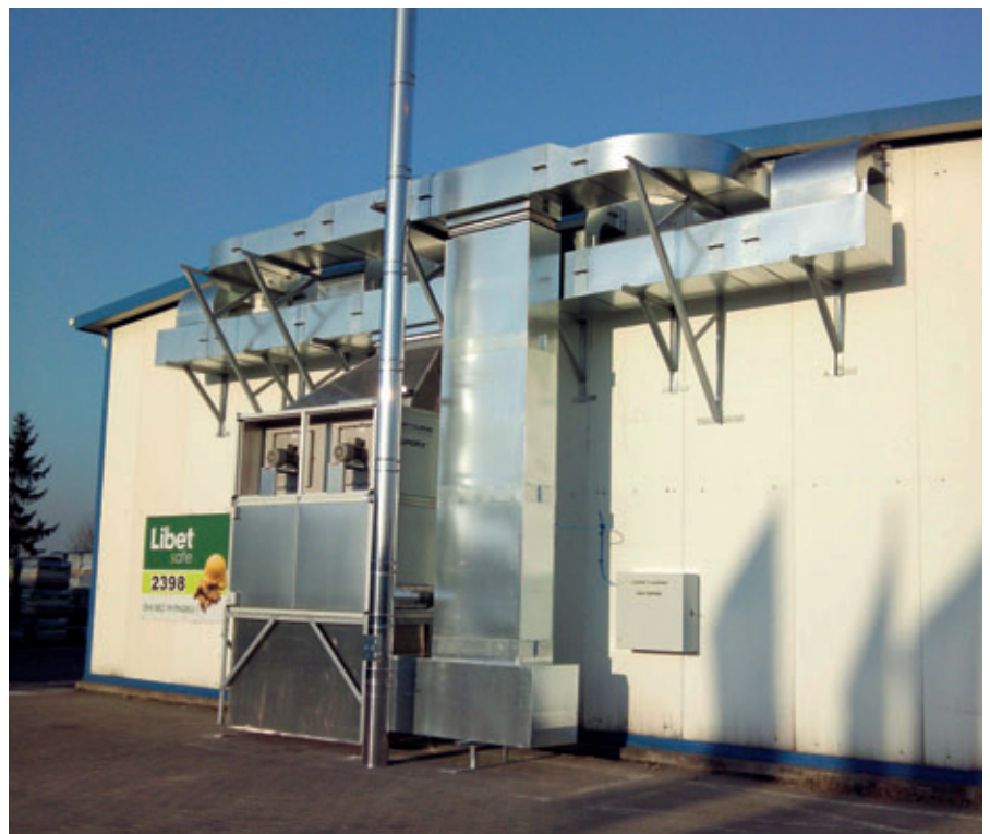
The complete Quadrix® system was installed at the rear of the insulated curing chamber. This system was equipped with an enclosure before the winter. Insulated ducts reduce the energy requirement. The heater and the flue are lined on the inside with high-quality stainless steel.
