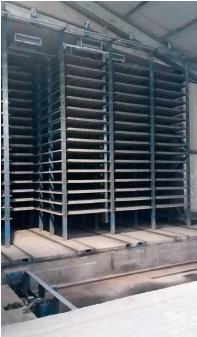
The supply air duct above corridor no. 7 controls the warm air in the finger car area to keep the temperature constant to \pm 1\text{ }^{\circ}\text{C} in the entire chamber system, even in the finger car area.
