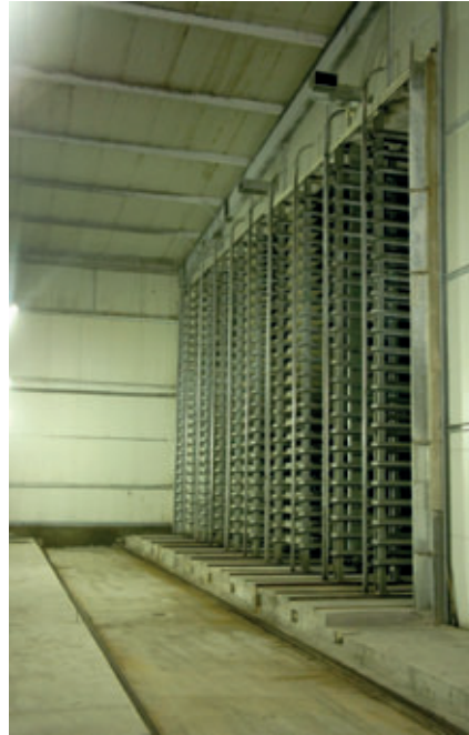
2015 – Single Atmosphere Curing with transfer car area and open rack area curing at 30°C and 90 % rH.
