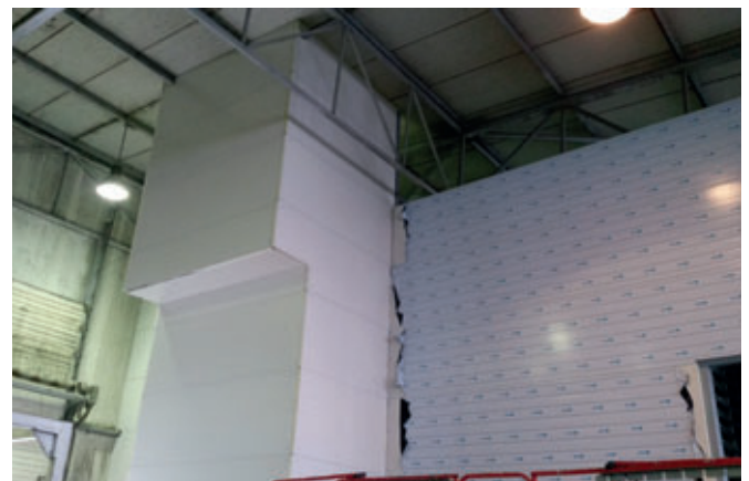
Installation of insulation panels around the elevator prior to completion of trim work. The insulation of the wall requires a total of 5 working days.
