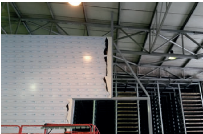
Installation of steel frame and insulation panels for insulation wall between the production and curing areas.
