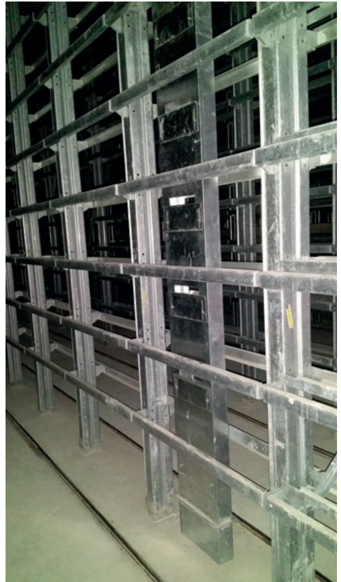
One of 15 air supply drops located throughout the chamber. Each drop includes adjustable air outlets at each level for a completely consistent atmosphere with consistent low air velocity in order to prevent moisture evaporation from the concrete surface.
