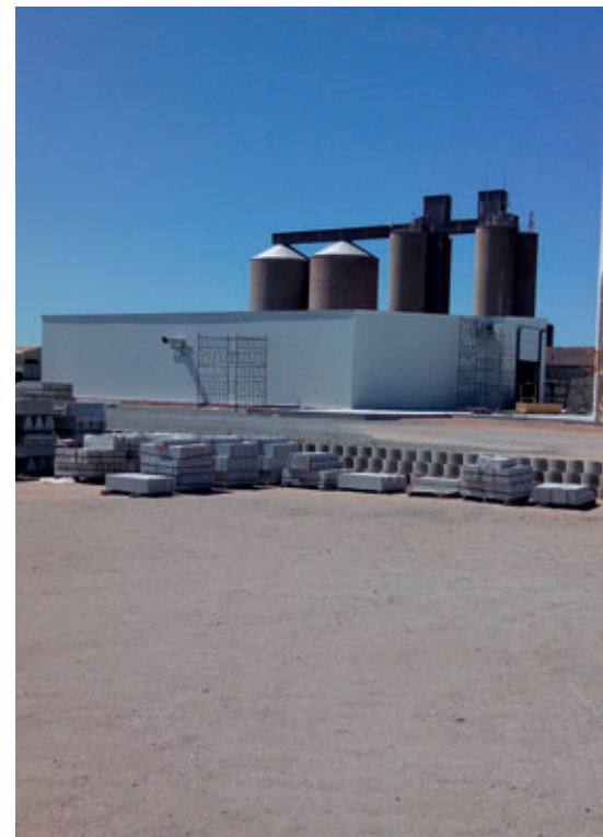
Curing rack exterior insulation, steel transport rails, fast operating door and air circulation system completed.
