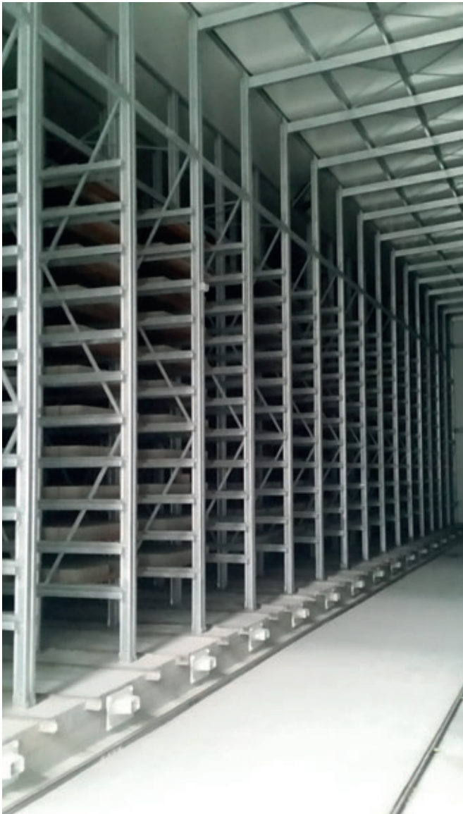
Single Atmosphere Curing Chamber with consistent temperature and relative humidity, no condensation on the ceiling, floor, steel racks or rails. Insulation, air circulation and humidity control is key in proving this type of curing/production environment.
