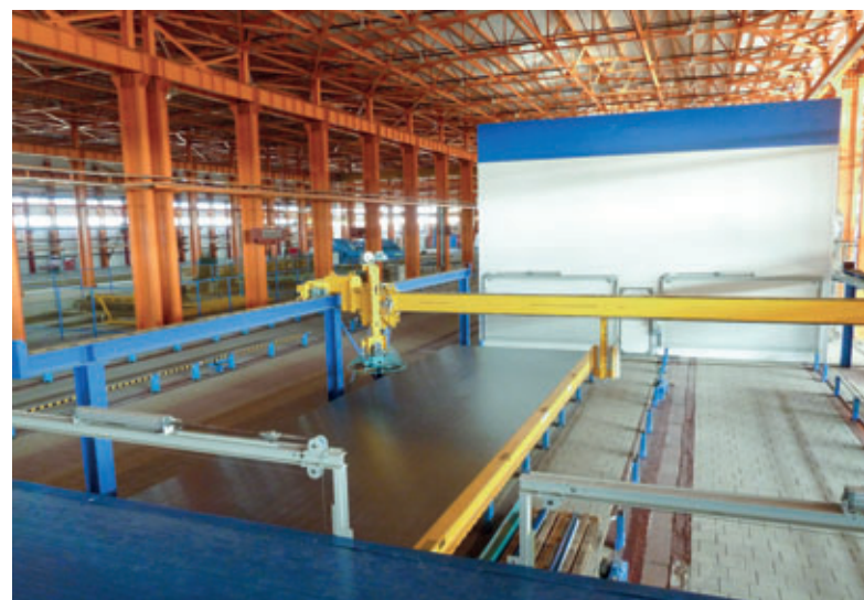
Following a pre-curing phase, the sandwich wall is smoothed with a power trowel.
