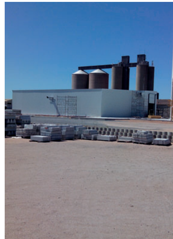
Curing rack exterior insulation, steel transport rails, fast operating door and air circulation system completed.
